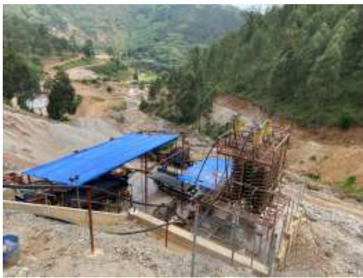
New upgrading plant at the tunnel
